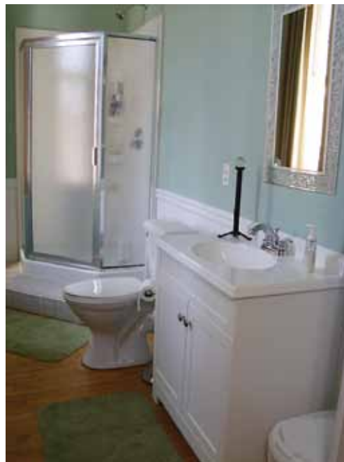
St. Paul's Church, Mount Vernon, and Harcourt Parish, Gambier teamed up to build this bathroom for the evening shelter at St. Paul's.
