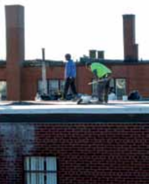
◀ Construction workers laying a new flat roof over Church of the Ascension, Lakewood's parish hall. The roof was completed in November 2014.
