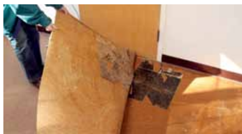
Renovation has commenced at St. Paul's, Maumee: asbestos tainted tile is removed and a section of the building is taped off in preparation for updates. >
