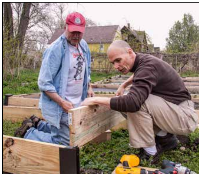
Trinity members Steve Roberts and Bill DiTirro work together to construct new raised beds.
